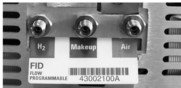
Figure 10 Gas line connections
